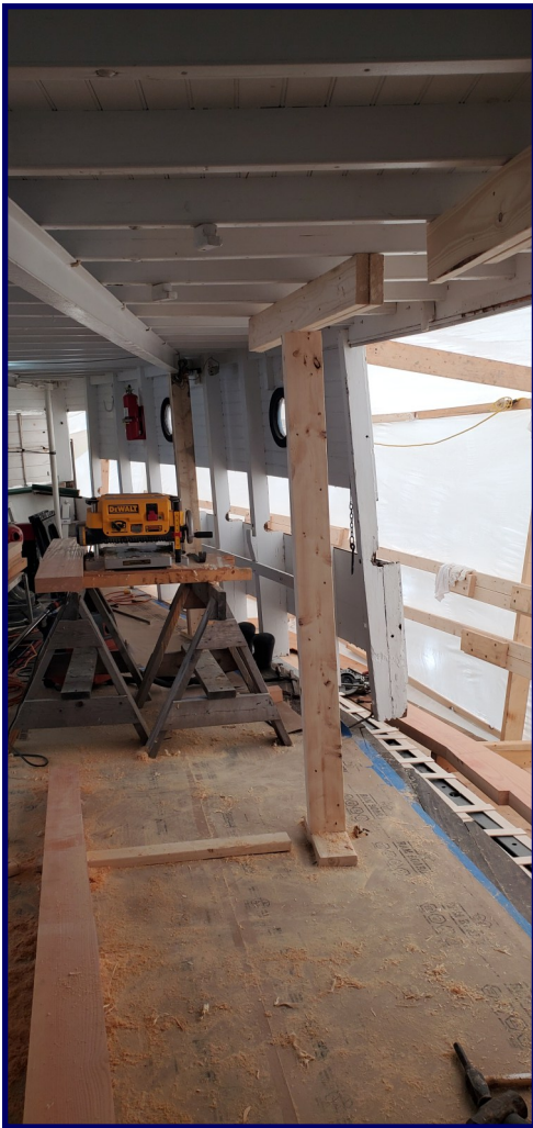
Starboard bow view. Note missing side strakes and new covering boards at lower right corner.
