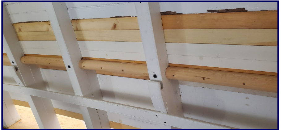
New Green Rail and side strakes. Note that some of the original side strakes were re-installed.
