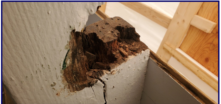
This is the edge where the green rail meets the cargo bay door. The replacement can be seen on the previous page in the lower right hand photo.
