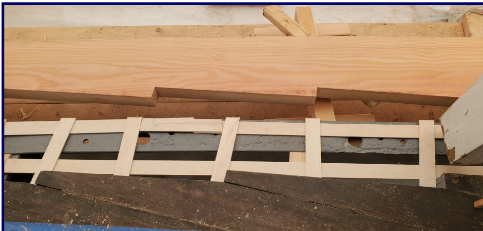
Brand new covering boards! The lattice at the bottom is the scaffold.
