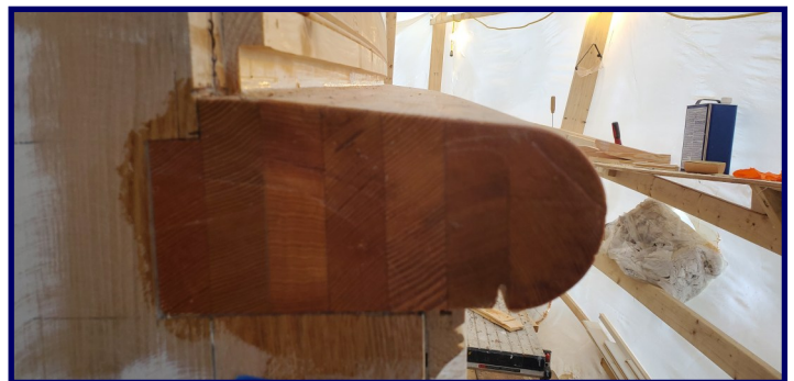
The new green rail. Note the drip groove on the underside to the right and the cambered upper surface.
